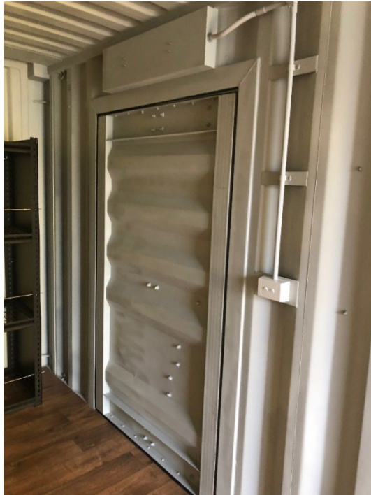
Figure 8 – Front Door (from inside container)
