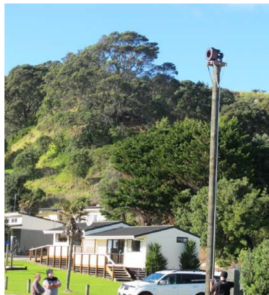
Ian Castles of Opotiki District Council overseeing the installation of the siren at Ōhiwa Holiday Camp.
