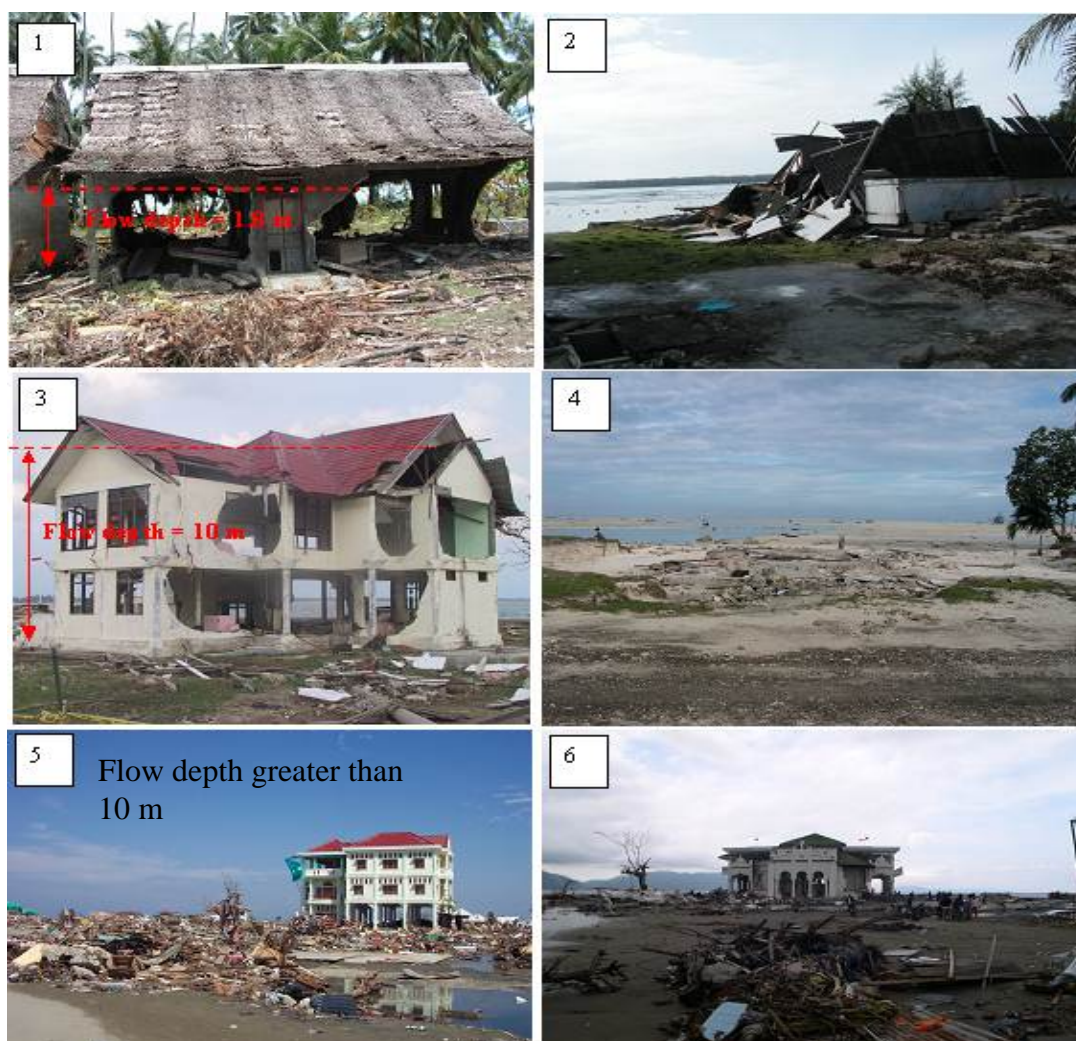
Figure 4 Typical damage to different types of houses due to tsunami with different flow depths in Banda Aceh and Nias Island after the 26 December 2004 event. Most of the 3 storey reinforced concrete structures survived the tsunami with flow depths greater than 10m (photo 5 and 6) whereas other buildings which surrounded these were completely wiped out. With this flow depth, no sheltering effects from the buildings or trees reduced the tsunami impact. A simple house with a palm tree roof was resistant to the earthquake shaking (photo 1) when compared to the neighbouring concrete house (photo 2). However, this house suffered damage from the tsunami with a flow depth of 1.8 m or half of the height of the house (Modified from: Prasetya et al. 2008).
