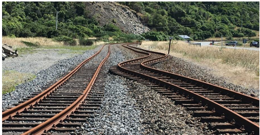
Rail Lines following Kaikōura Earthquake, 2016
