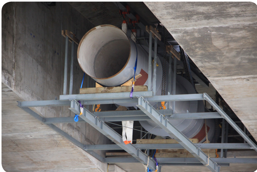
Above: New watermain under construction beneath Mangere Bridge, Auckland. Collaboration is often required between different infrastructure owners when new construction or maintenance are planned. Credit: Watercare Services Ltd
