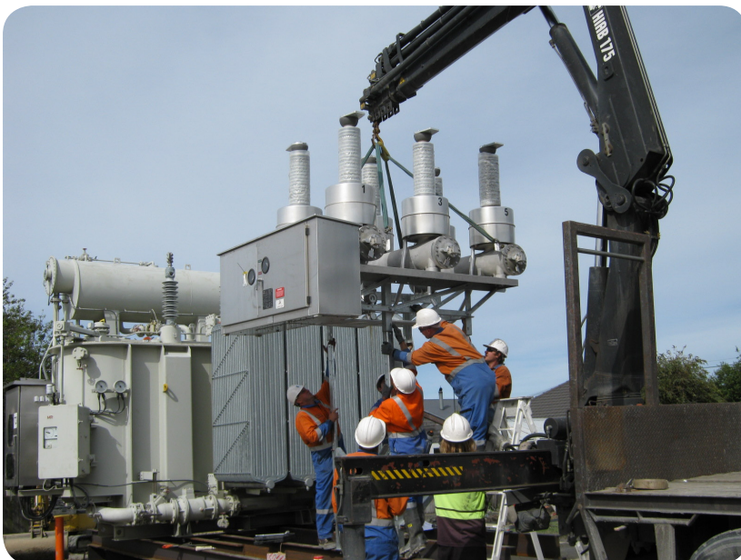
Left: Installation of a temporary transformer at the New Brighton substation, Christchurch, following the February 2011 earthquake. An emergency 66kV overhead line was also quickly built to supply the area. Credit: Orion New Zealand.
