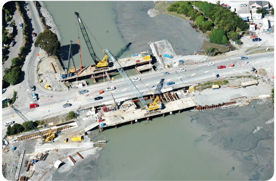
Above: Ferrymead Bridge, Christchurch, under redevelopment. This photo, taken soon after the February 2011 earthquake, shows extensive riverbank damage and liquefaction in the area. Credit: H.A. Cowan.
