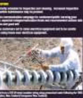
Insulator flashover can be caused by a number of factors, including:
