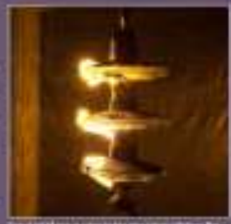
Insulator flashover can be caused by a number of factors, including:
