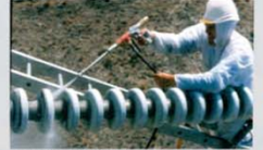
Ash is cleaned from a 110 kV horizontal insulator string using pressurized water following the 1996 Ruapehu eruption, New Zealand (Transpower New Zealand)
