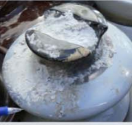
Ashfall covers a 33kV insulator following the May 2008 Chaiten eruption, Chile
