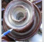
The underside of a 33kV insulator coated in ash, which led to flashover following ashfalls during the 2008 Chaiten eruption, Chile
