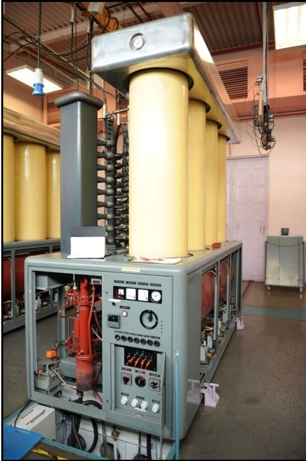
Pole 1 – Mercury Arc Valves (1965)
