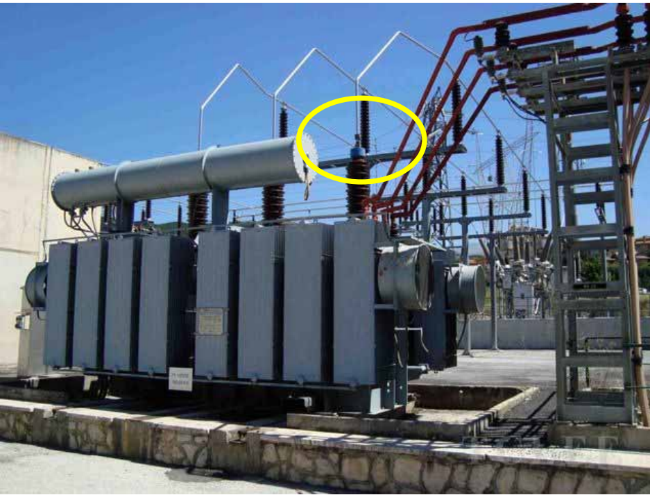
Damage to the rigid connection of a transformer
