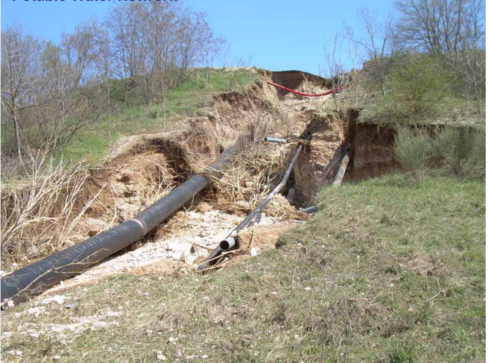
Joint slip-off in a main water network pipeline in Paganica.
