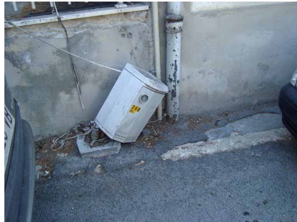
Damage to pedestal box
