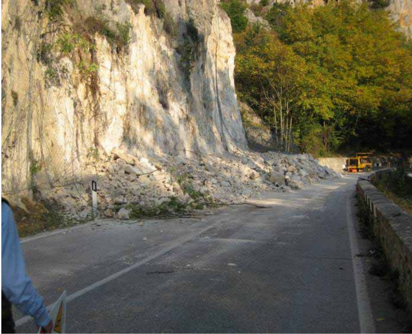
S.S. 5 “Tiburtina Valeria” rockfalls
