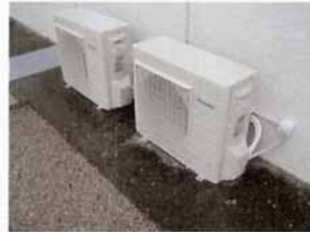
Airconditioning units restrained
