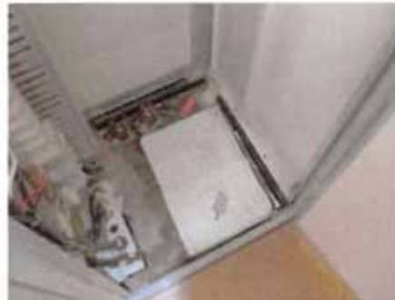
Typical cabinet hold down. Note manuals and paper should not generally be left in cabinets due to potential fire hazard
