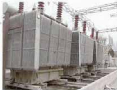
Older single phase transformers well restrained
