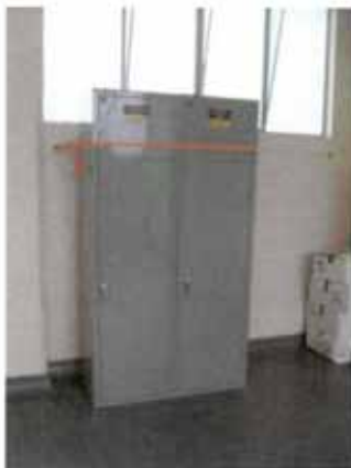
Restrained cabinet good practice
