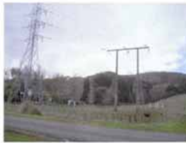
Termination tower and H poles
