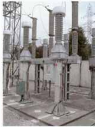
VT's on sturdy pipe stands
