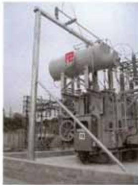
Newer type RHS and pipe gantry
