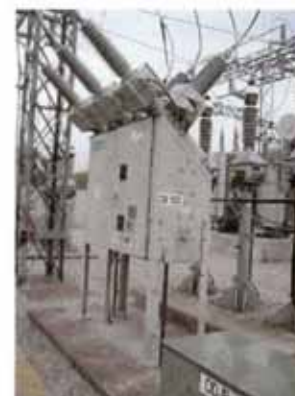
Three phase CB inside cabinet on cantilevered legs
