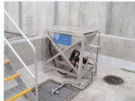
Oil Separator unit well restrained
