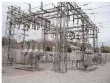
33 kV area showing gantry and switchgear
