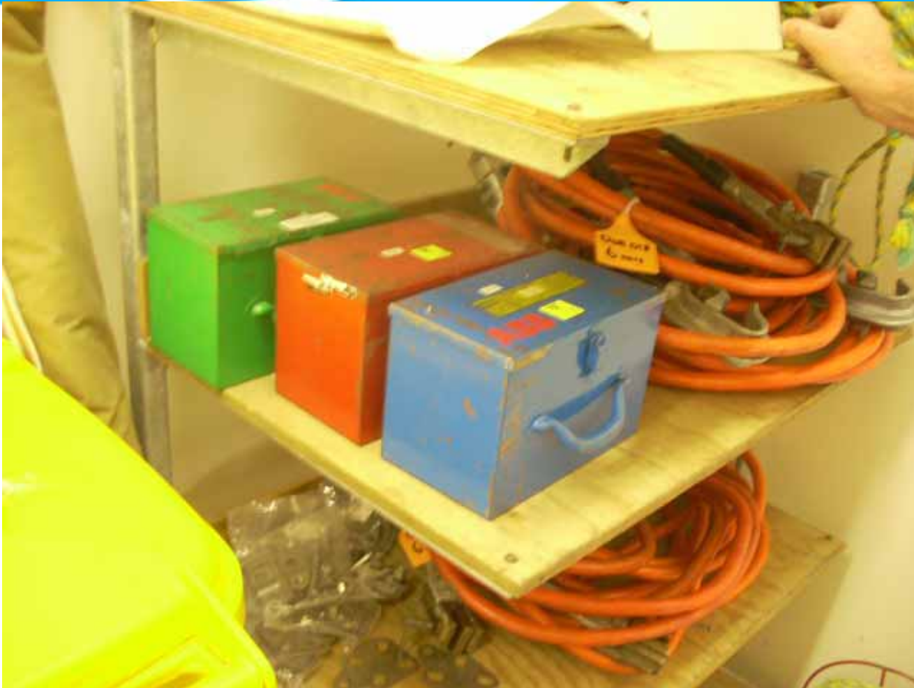
Equipment vulnerable on shelving
