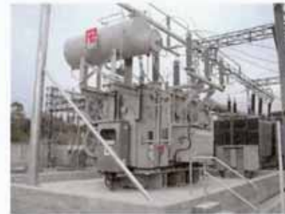
Newer three phase transformer well bolted down
