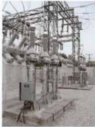
VT's on sturdy pipe stands
