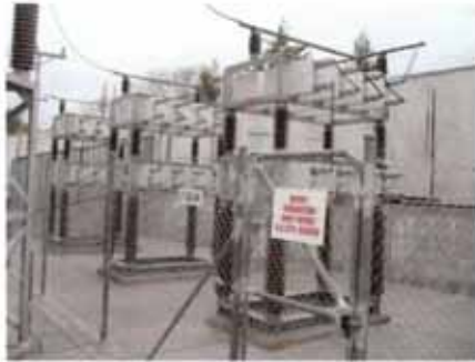
Capacitor banks on post insulators
