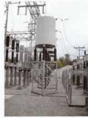
Reactors on lattice stands
