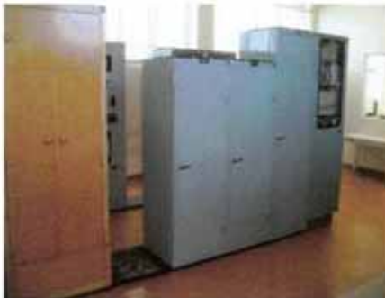
Cabinets in the relay room
