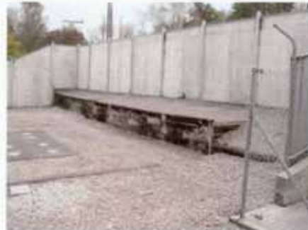
Retaining wall has moved in the past and should be monitored
