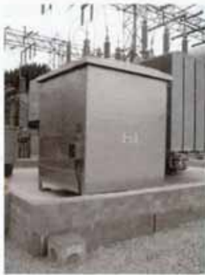
Neutral Earthing Resistor bolted down to transformer pad
