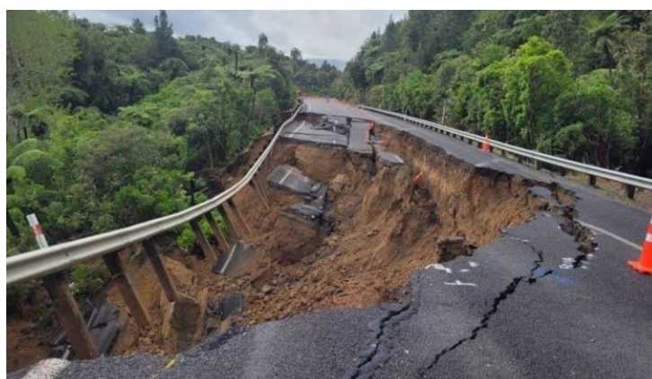
Figure 1-4: North Island Road Damage
